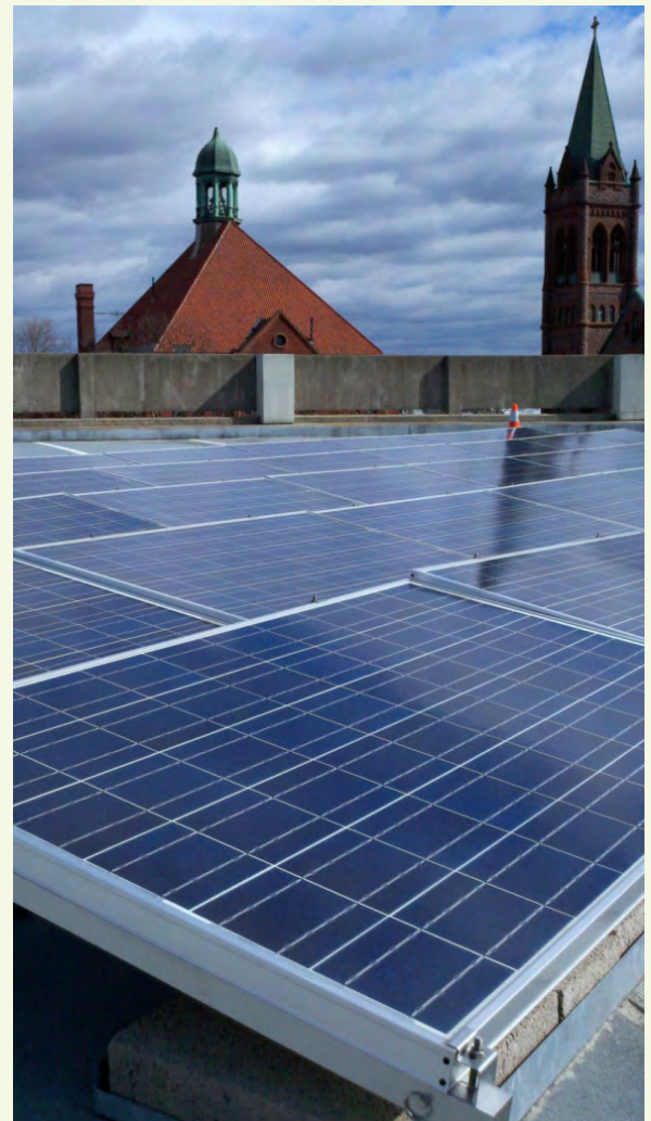
Caption: 30 kW Solar Panels on Fort Stanwix Parking Garage, Rome, Oneida County
