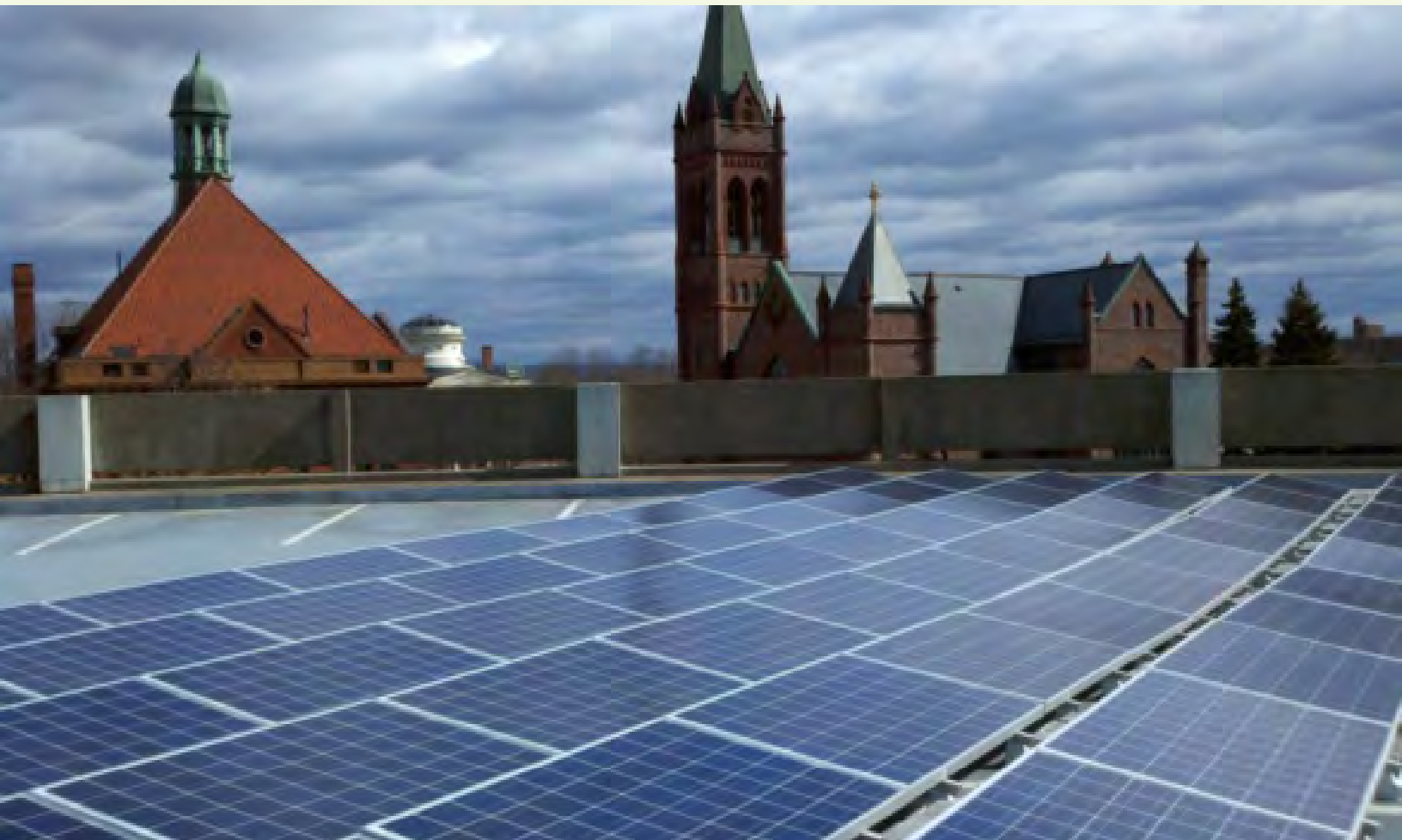
30 kW Solar Panels on Fort Stanwix Parking Garage, Rome, Oneida County
