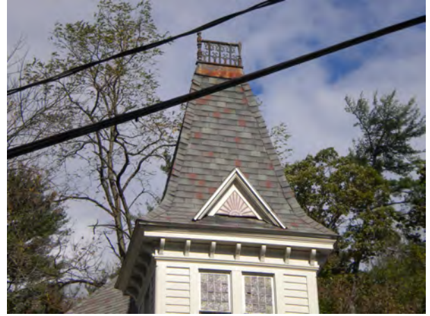
House, turret detail, damaged cresting, facing NE
