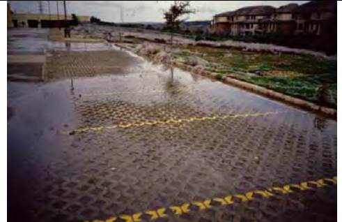
Water standing on the parking surface 48 to 72 hours after a storm is an indication of clogging. Snow piles at the edge of the photo point to possible clogging from winter sanding or plowing.
