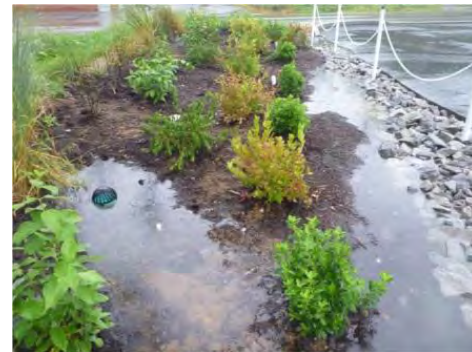
Water is preferentially ponding only at one end of the bioretention because the surface is not flat.
